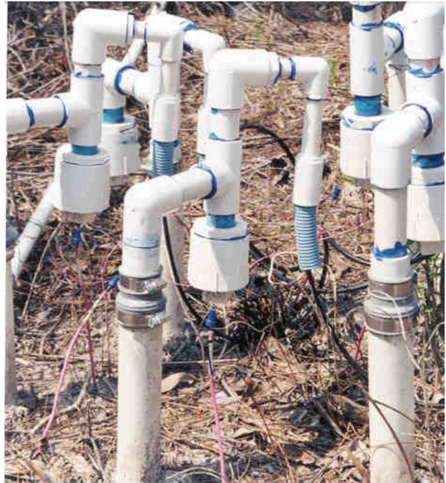
Figure 5.—Proper installation and monitoring of equipment as described in the Hydric Soil Technical Standard is required to collect data regarding proposed additions, deletions, or other changes to the hydric soil indicators.
